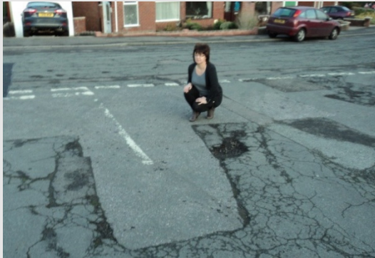
Despite some welcome investment there are still problems with roads and pavements all over RCT, such as here in Heol Deg
